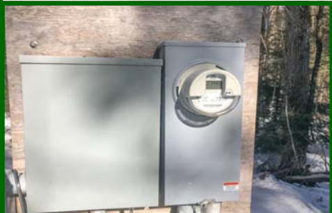
Electric Service to Property
