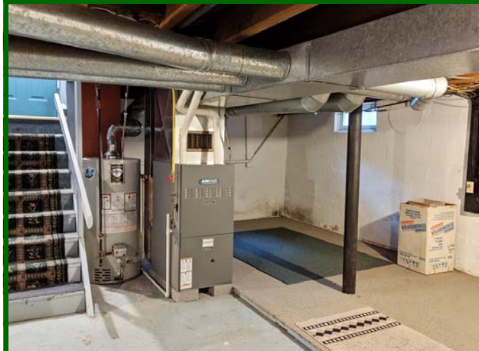
Furnace & Hot Water Heater
